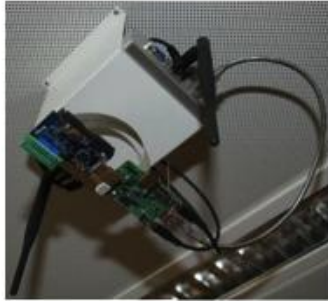
Transmitter Wi-Fi Node
